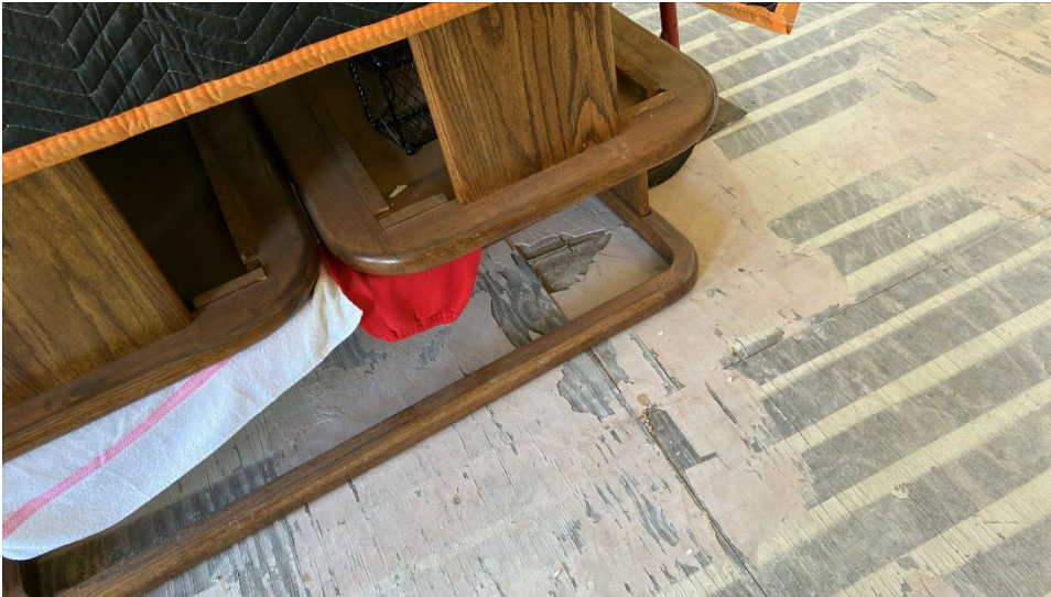
Living room area subfloor ?
