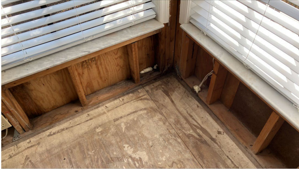
Dining room area, rotted, framing
