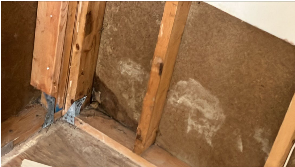
Rotted wood sheathing kitchen area
