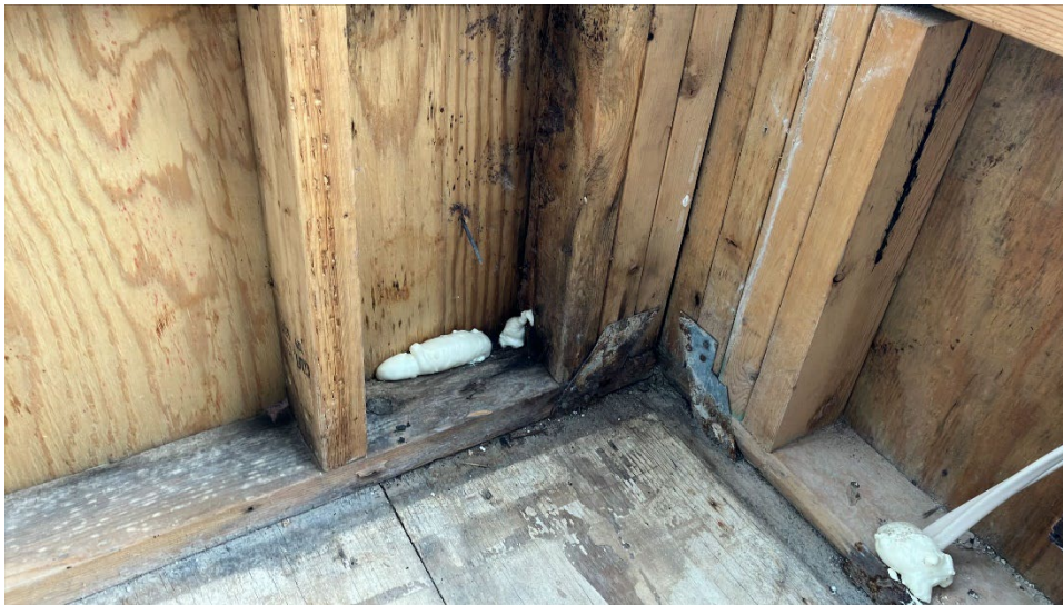
Dining room area, rotting subfloor
