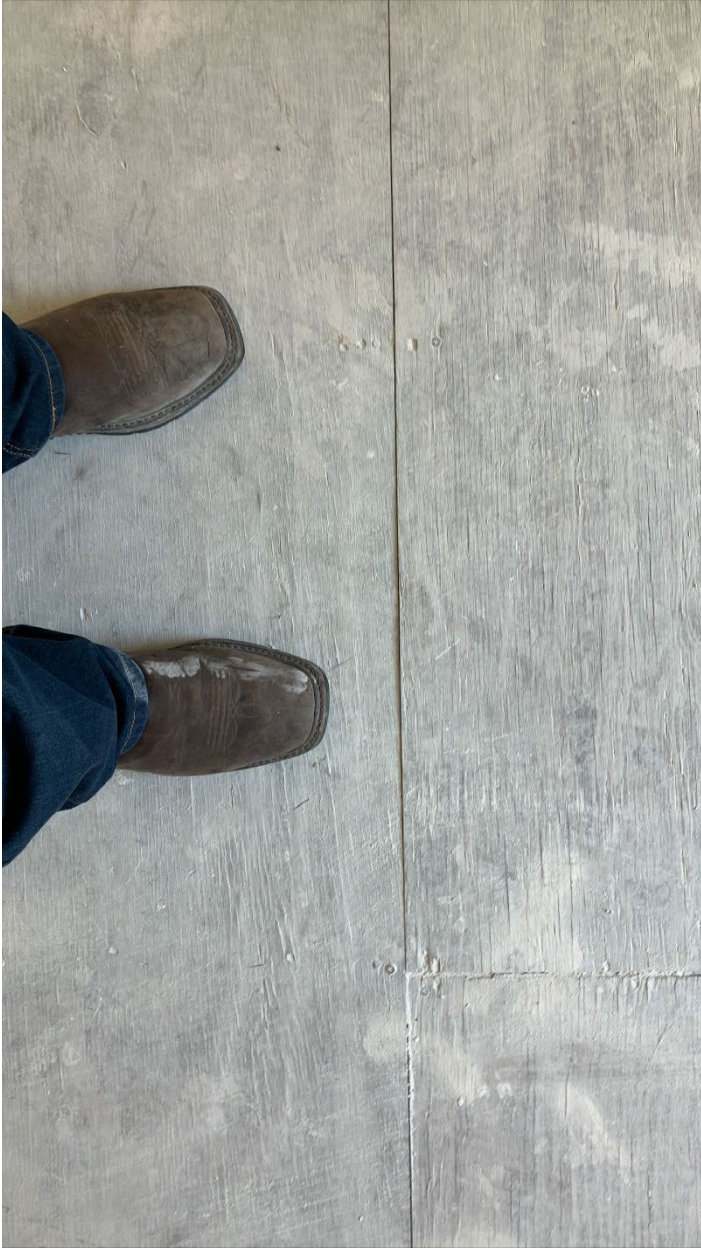
Subfloor in guest bedroom loose
