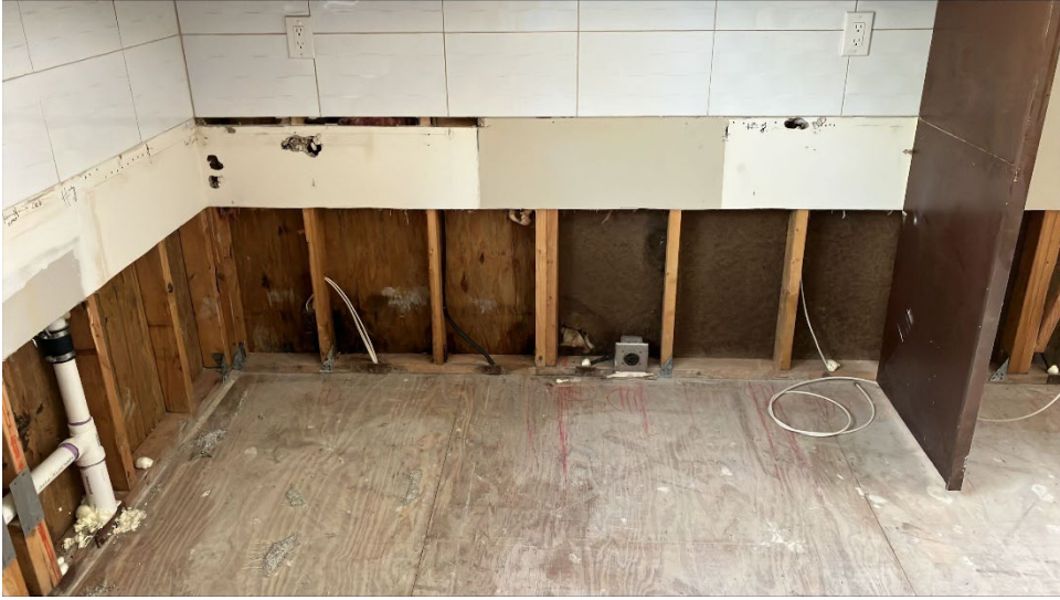
Kitchen, rotten wood sheeting
