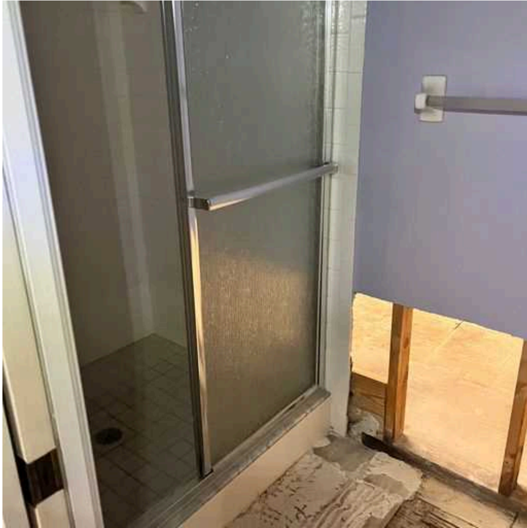
6 Main Level/Master shower - 4- Master Shower
