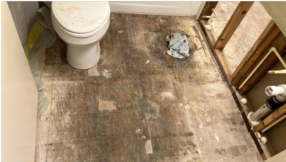
Guest bathroom, subfloor
