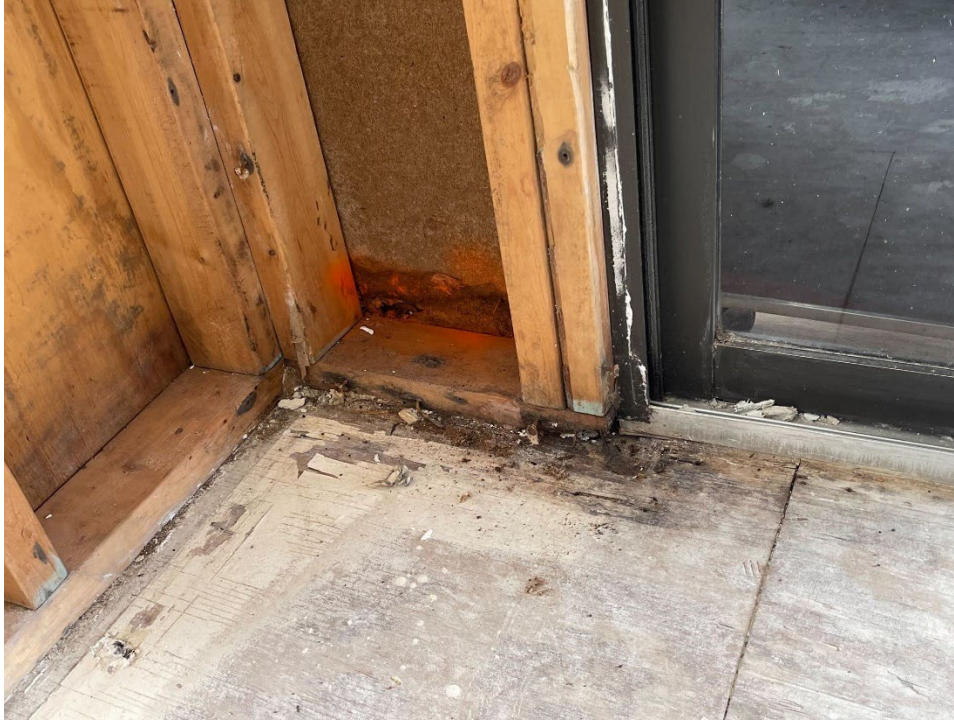
Left and right side of the floor and wood sheeting next to sliding glass door and several other spots in master bedroom.
