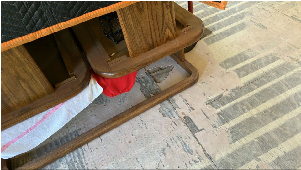
Living room area subfloor ?
