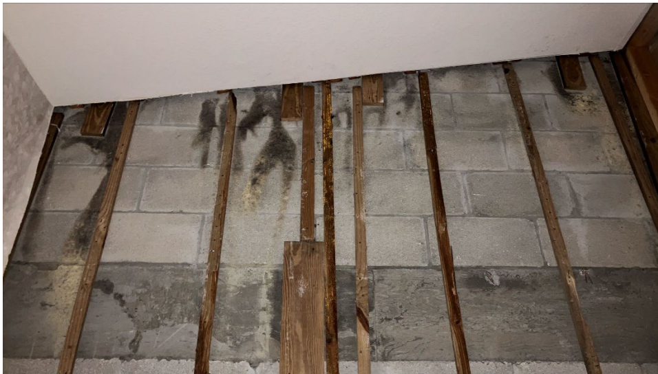
Master bathroom, potentially mold on cinder blocks
