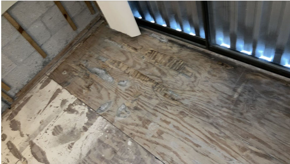
Subfloor in front of sliding glass door, master bed
